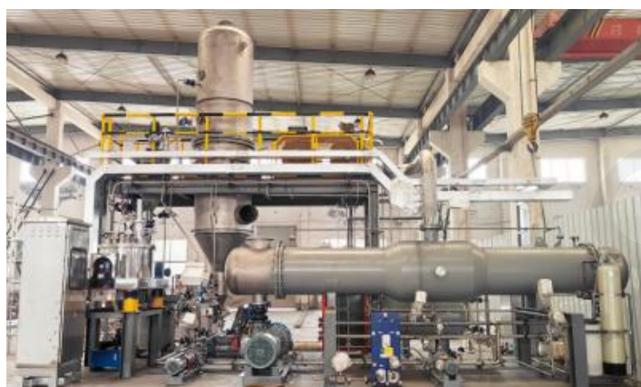
Skid Mounted Evaporator/System
